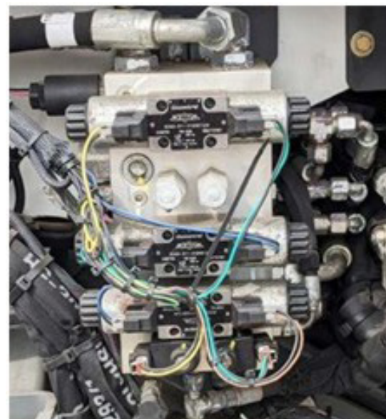
Fig. 68: Conveyor Hopper Manifold
