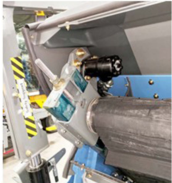
Fig. 65: Conveyor Drive Motor
