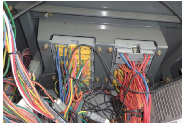
Fig. 1: Relay Panel Back
